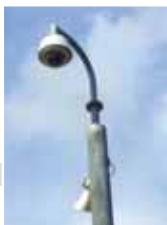
Traffic Control, Lights and Cameras
